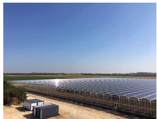
Technique Solaire's solutions include designing and installing photovoltaic greenhouses, optimizing land use and bringing value to farmers and local stakeholders.
