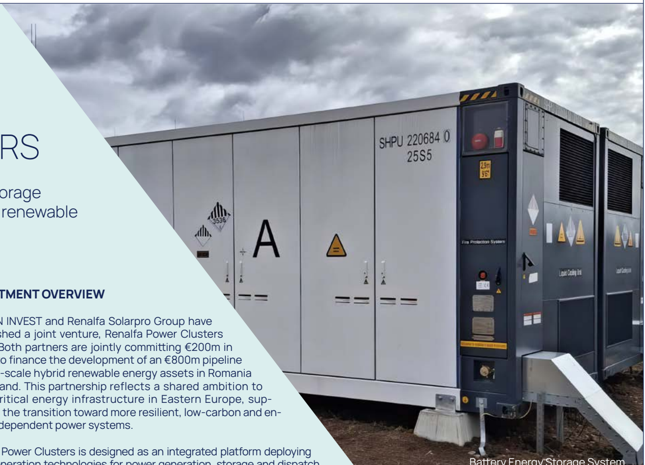
Battery Energy Storage System Renalfa Bulgaria
