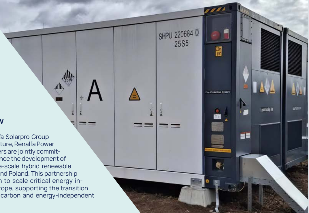
Battery Energy Storage System Renalfa Bulgaria
